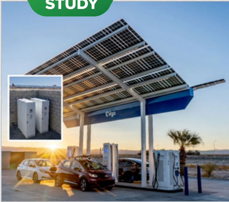
Figure 22: EVgo’s Charging Station in Baker, California
